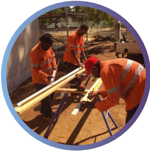
Jilkminggan community members (left to right) Stuart Yunupingu, Harry Albert and Matthew Conway at work building the community's new store.
